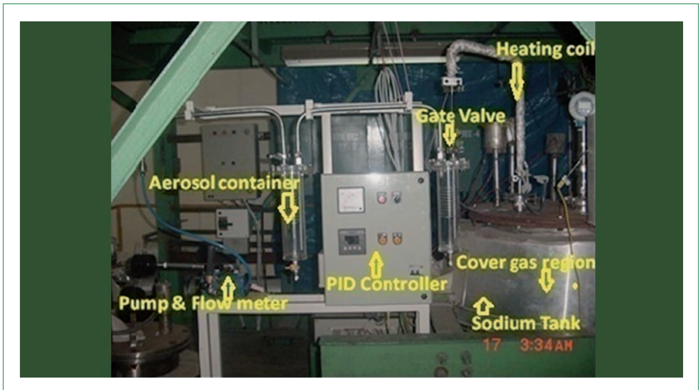
Figure 1: Photograph of aerosol sampling system integrated with test pot-1 of SILVERINA loop
