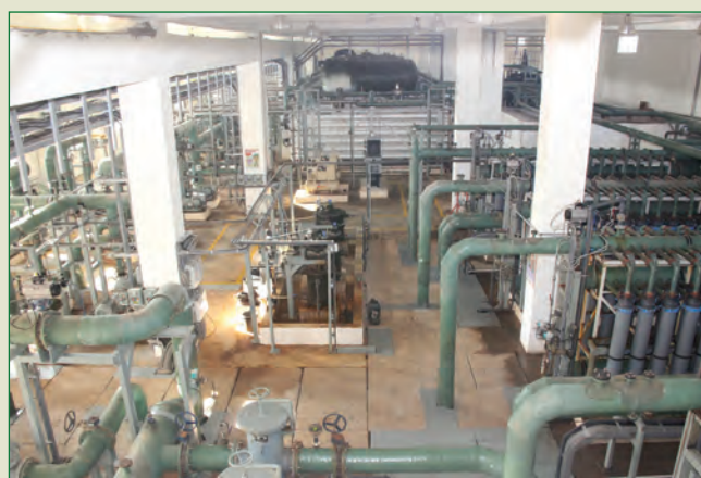
Piping and Filtration Chambers
