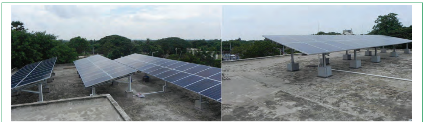
Figure 1: Solar Photovoltaic Panels at the roof top of ESG Annex Building
