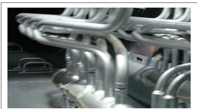
Figure 2 SG tubes in blanked condition
