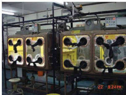
Figure 6: Mixer-settler facility used for flow sheet development studies with TiAP for fast reactor fuel reprocessing
