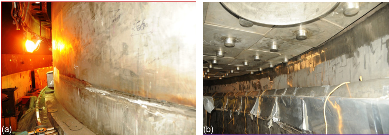
Fig. 2 Roof slab to main vessel weld joint (a) Outside view (b) Inside view
