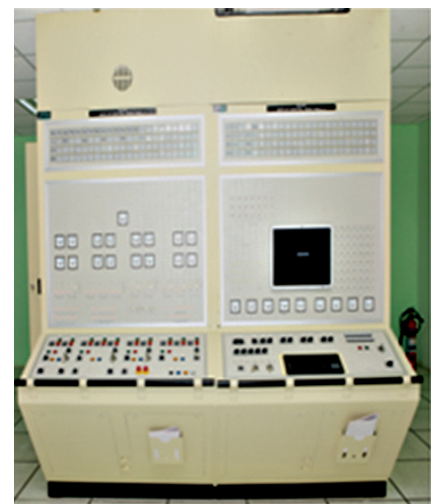
Fig. 4 Backup control room
