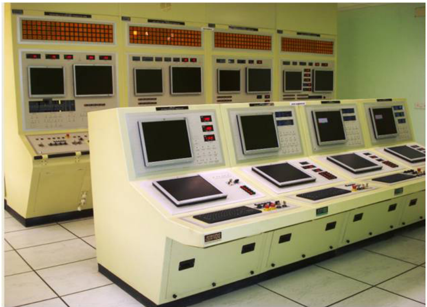
Fig. 3 Handling control room
