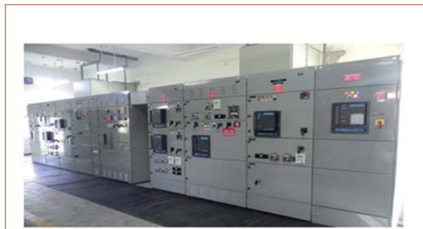
Fig. 2 PDC IX 415 V switchboard
