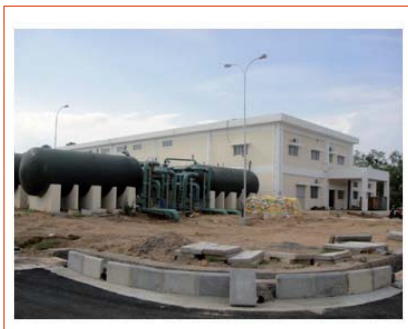
Fig. 1 Reverse osmosis plant
