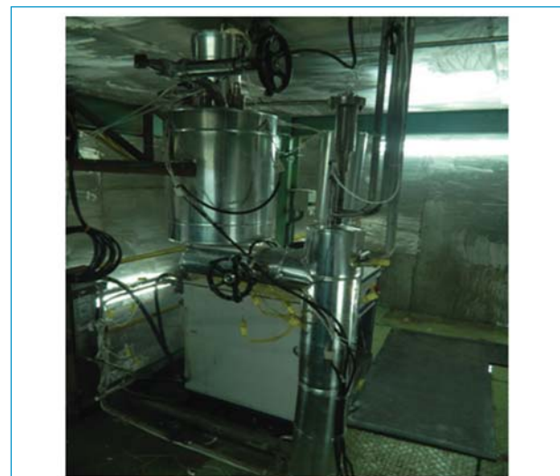
Fig. 2 Sodium filling system
