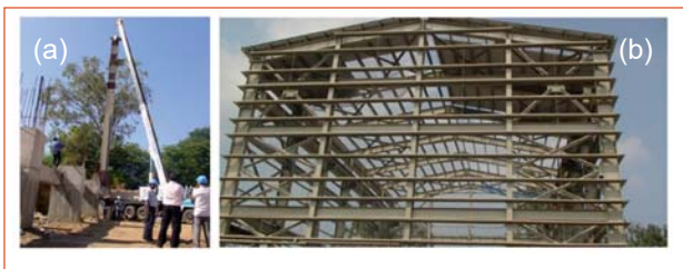
Fig. 1 (a) Embedment of steel column into concrete pedestal and (b) rigid frame using bolted connections
