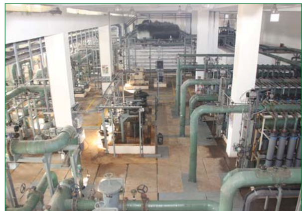
Piping and Filtration Chambers
