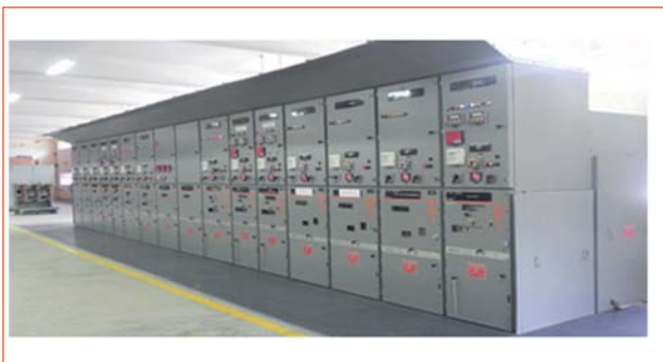
Fig. 1 PDC VIII 6.6 kV switchboard
