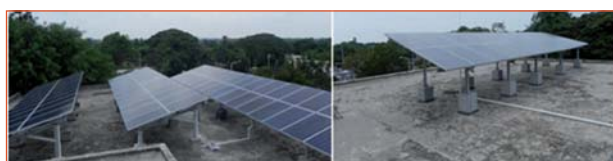
Fig. 1 Solar photovoltaic panels at the roof top of ESG annex building
