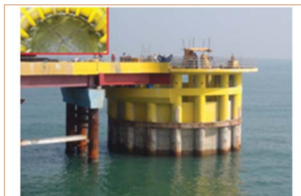
Fig. 3 Sea water intake structure
