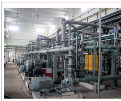
Fig. 2 Reverse osmosis feed water system
