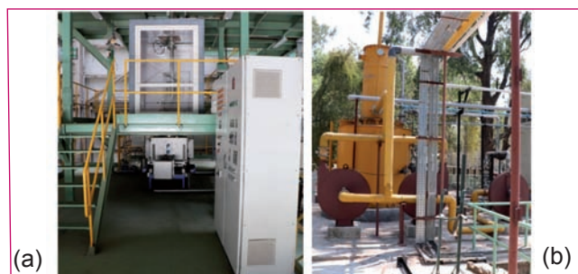
Fig. 2 (a)Chlorination vessel inside fume hood (b)chlorine scrubbing system
