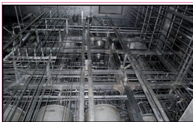
Fig. 1 Typical view of tanks and equipment with piping inside process cell
