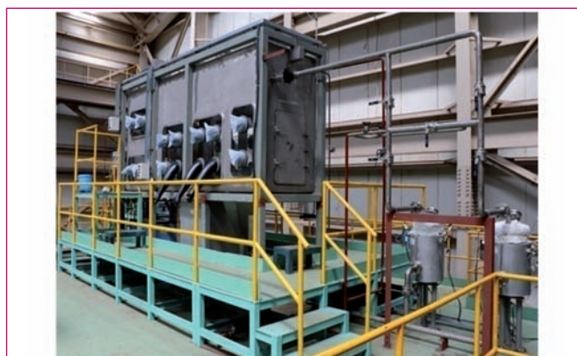
Fig. 1 Glove Box for salt mixing & vacuum drying
