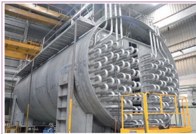
Fig. 2 Cooling coils and ballast tank
