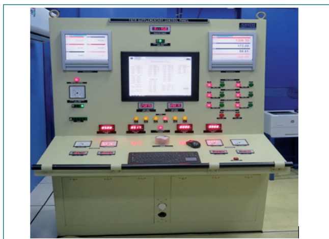
Fig. 1 Supplementary control panel installed in cabin
