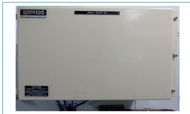
Fig. 2 Junction box installed in the field
