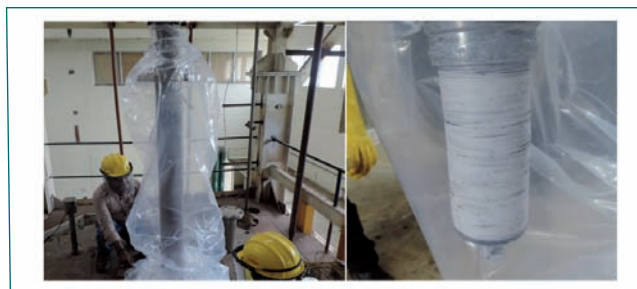
Fig. 2 Sodium wetted lower part and bellows
